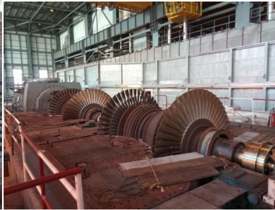
Both LP1 & LP2 turbine rotors placed condition
